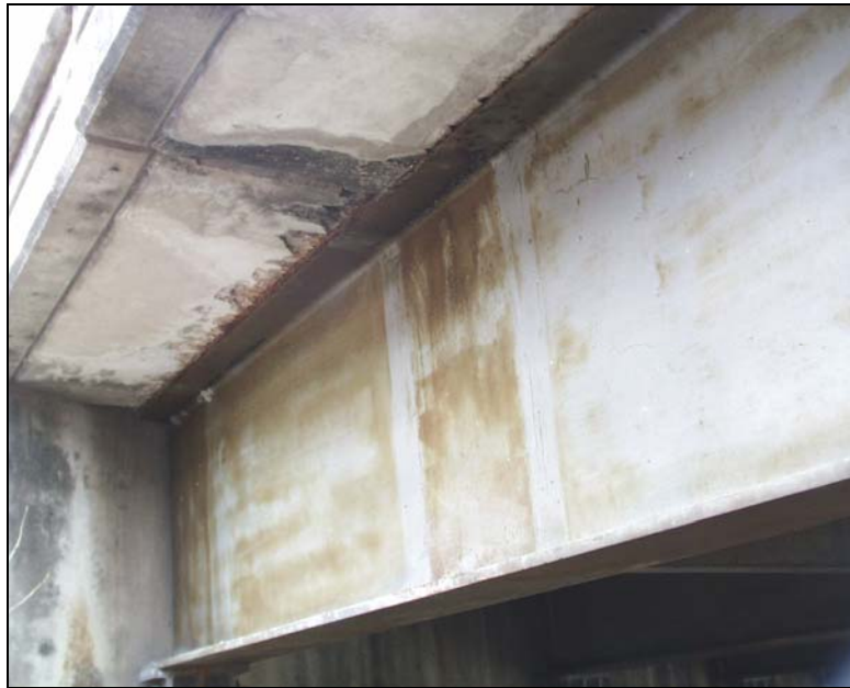
Figure 4.9: Spalling and rust at interface near abutment of Binz-Engleman Road bridge
