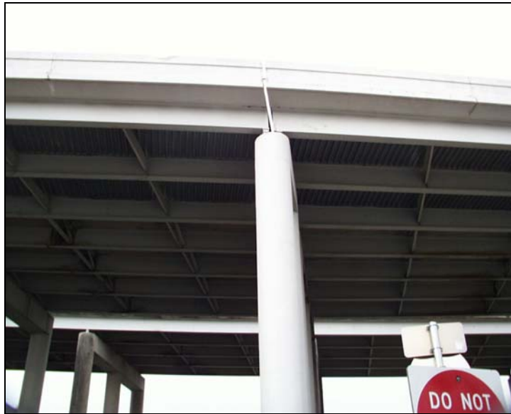
Figure 4.5: Expansion joint at an interior support on the Southern Pacific Railroad and FM 78 bridge
