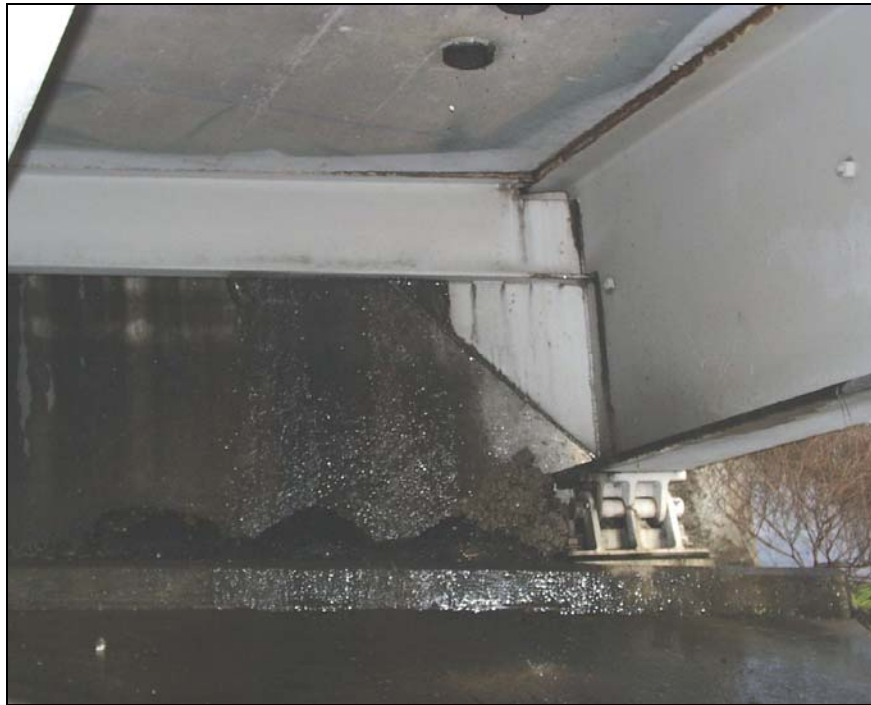
Figure 4.15: Expansion joint at abutment, rust, and pouring water on Southern Pacific Railroad and IH-35 Northbound bridge
