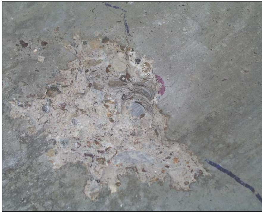
Figure 6.28: WEDGB01 failure with spalled concrete
