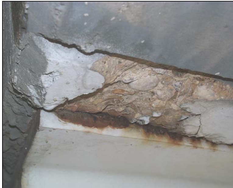
Figure 4.12: Close-up of spalling and rust shown in Figure 4.11
