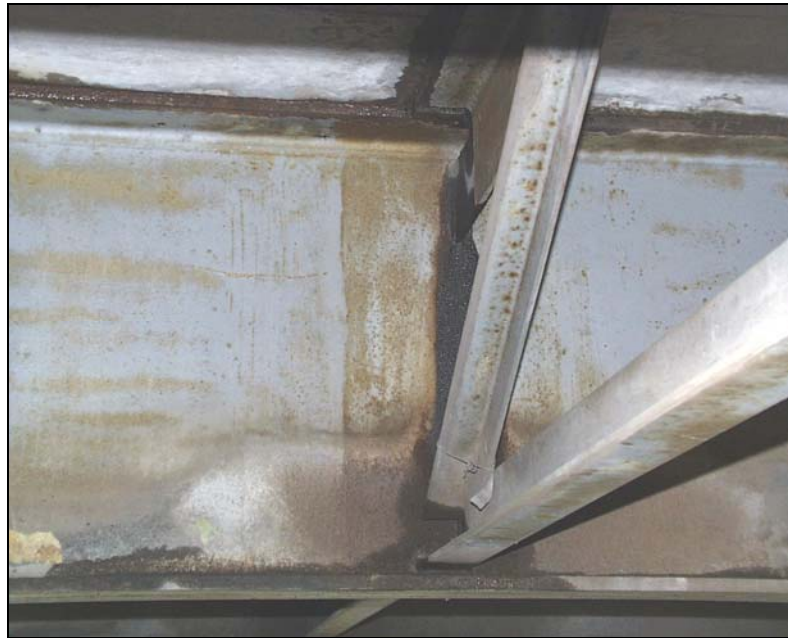
Figure 4.14: Rust at lateral bracing on Binz-Engleman Road bridge
