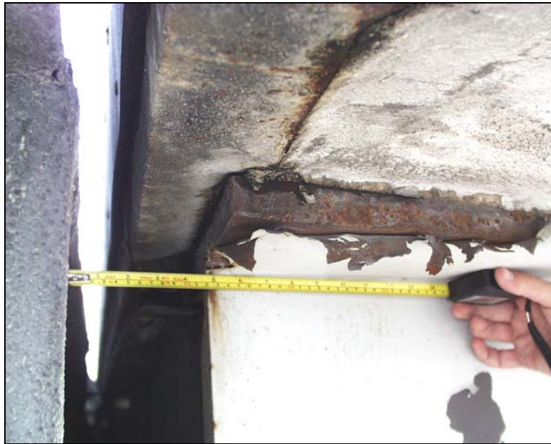
Figure 4.10: Expansion joint gap, rust at interface, and peeling paint near abutment of Walzem Road/FM 1976 bridge
