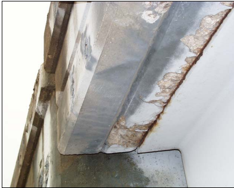
Figure 4.11: Extensive spalling and rust at interface of the slab and girder near the abutment of Southern Pacific Railroad and IH-35 Northbound bridge
