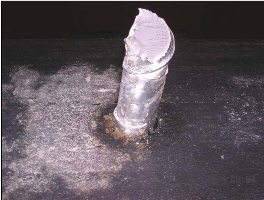
Figure 6.24: WEDGS failure with protruding sheath
