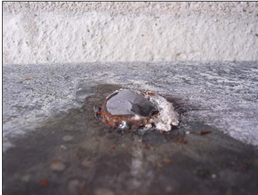
Figure 6.2: Typical failure of Welded Stud above the weld pool
