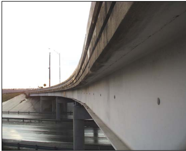
Figure 4.4: Continuous structure over interior supports on Southern Pacific Railroad and IH-35 Northbound bridge
