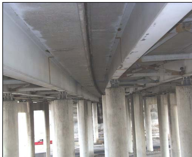
Figure 4.17: Typical conditions on underside of Honeysuckle Lane bridge
