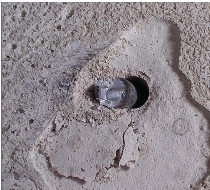
Figure 6.8: Typical failure of Cast-In-Place Welded Stud, particular specimen with air void
