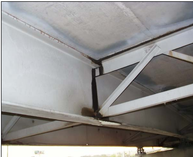
Figure 4.13: Extensive rust at lateral bracing on Southern Pacific Railroad and IH-35 Northbound bridge
